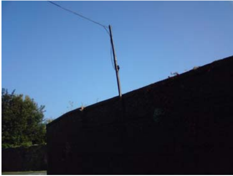
Fig 6. Distribution pole and cable box
