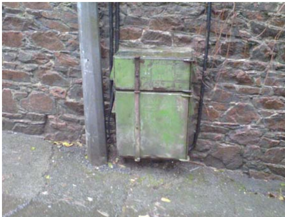
Fig 11. Local distribution amplifier
