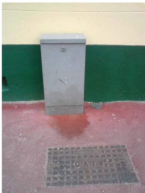
Fig 14. Jersey Cable distribution amplifier and manhole cover
