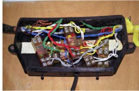
Fig 1. Distribution box showing Baluns
