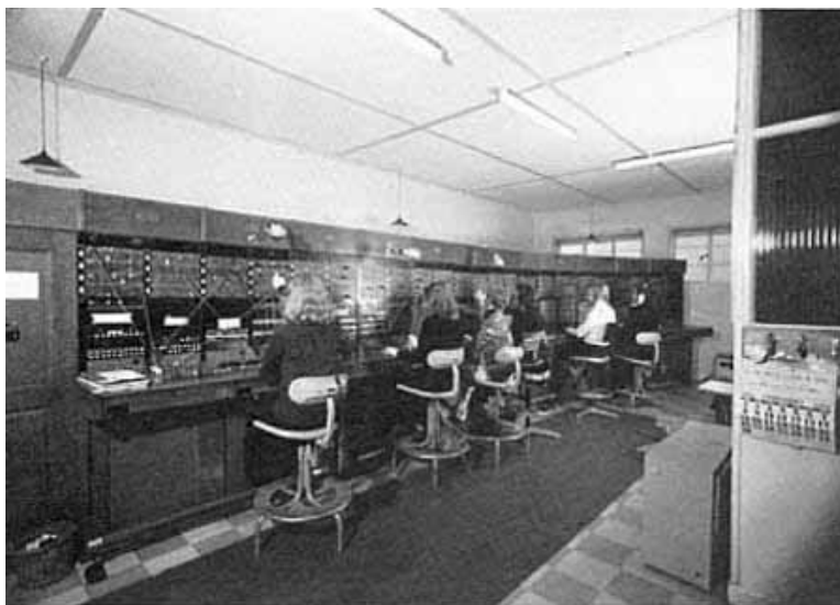
The Jersey West manual exchange switchroom showing the Ericsson of Beeston board.
